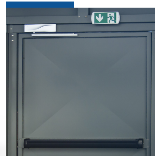
Mechanical panic bar, door locker and emergency lighting
